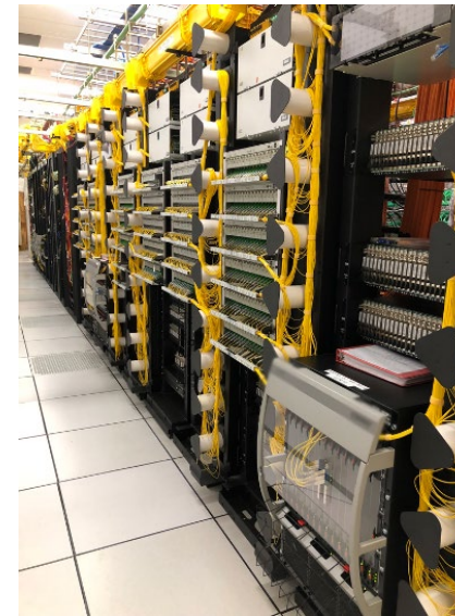
Legacy: Pod = 96 service groups 5 Racks
