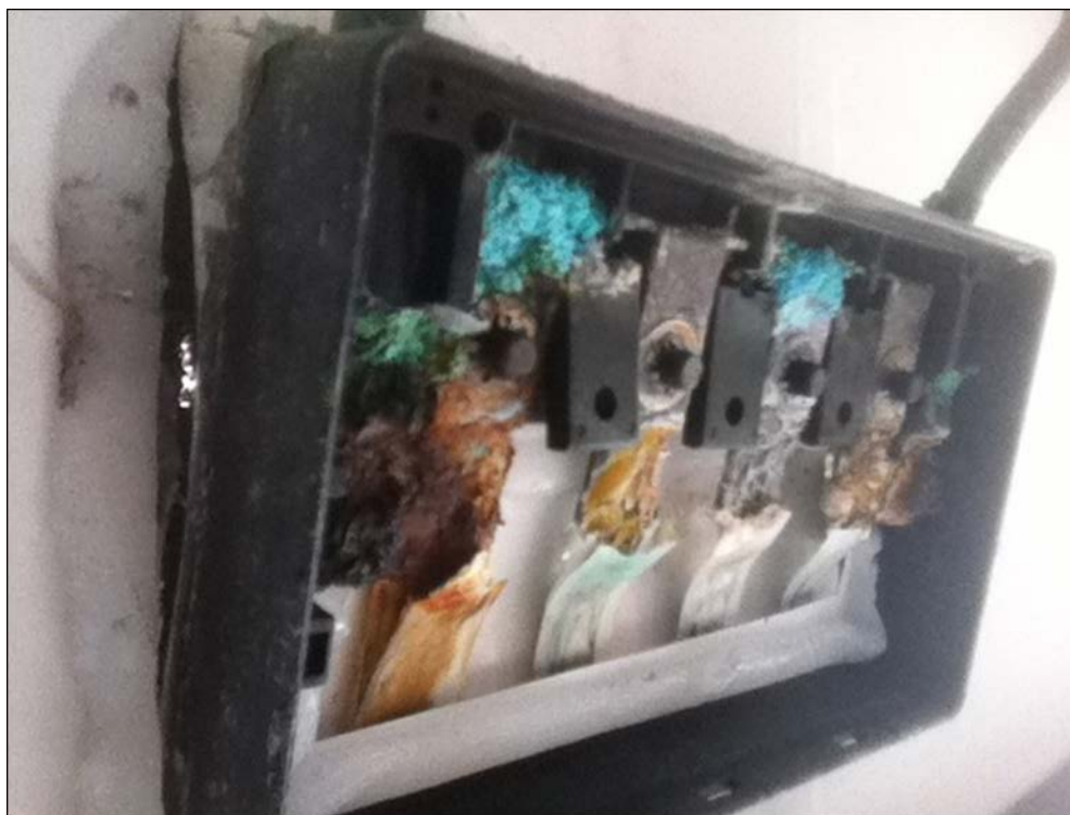
Figure 14 -Failed Junction Box
