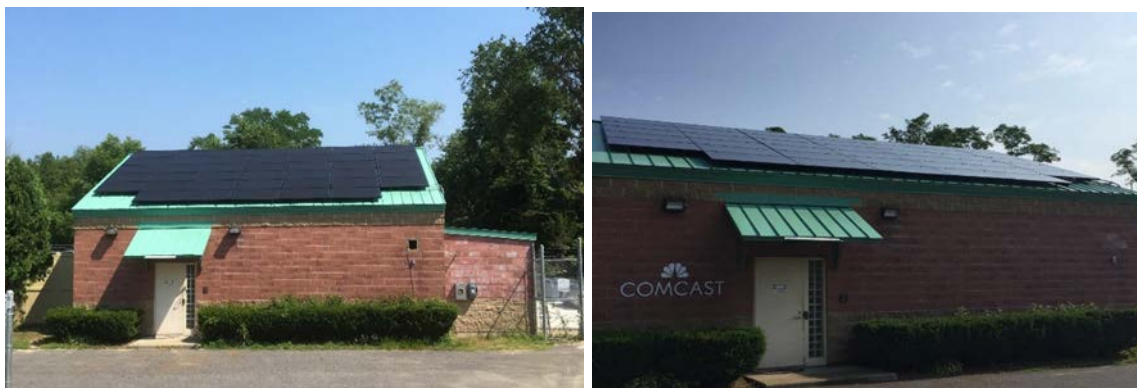
Figure 1 - Solar PV installed at Headend
