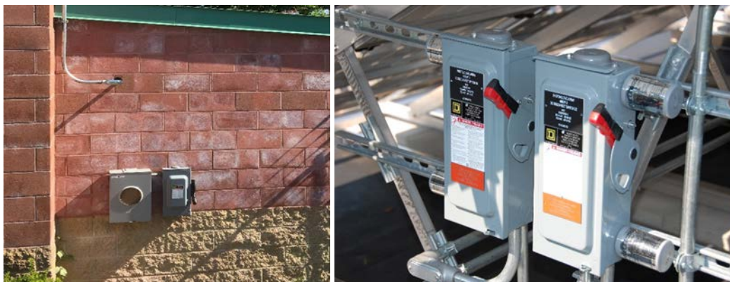
Figure 17 - Meter and Disconnects
